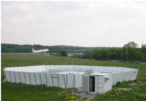
Figure 3. WTR/RASS at Frankfurt airport
